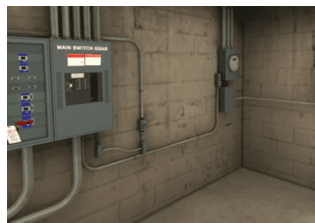
Lockout Tagout: Electrical room
